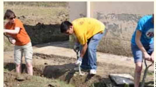
Shelby Mills (left), Michael Santos, and Kristen Schwindt work hard digging a two-foot-deep trench in preparation for a cement wall.
